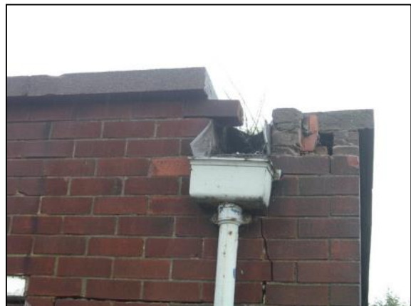
Photo 41: Damage to wall & roof
