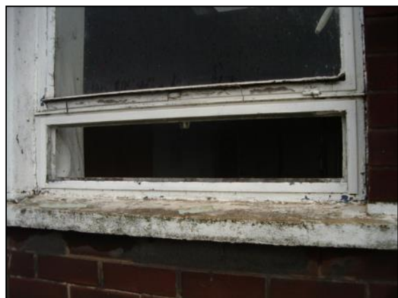
Photo 43: Window with missing pane
