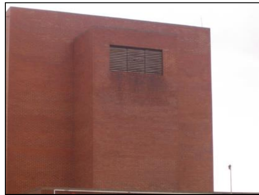
Photo 57: Close up of ventilation panel
