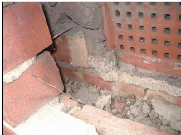
Photo 31: Wall cavity visible
